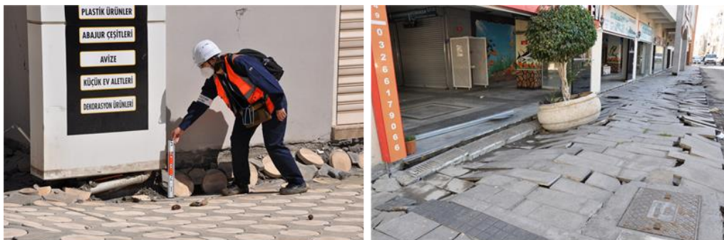
Figure 6. Settlement of buildings due to soil liquefaction
