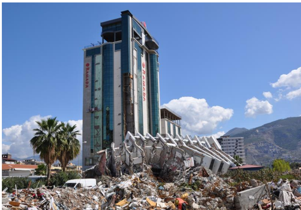
Figure 4. Collapsed building located in the former marshland – near Hotel Ramada
