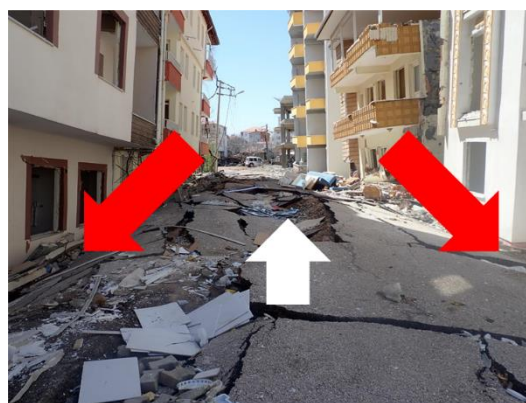
Figure 18. Road uplift and settlement / tilting damage to buildings on either side of the road
