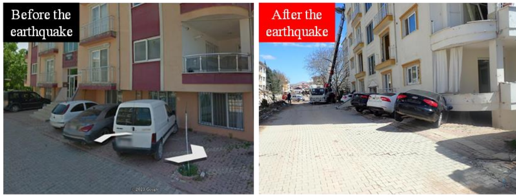
Figure 17. Building suffered from subsidence of about 1.5 m – before and after the earthquake
