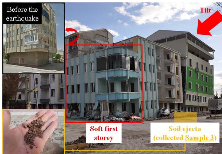
19. Structural damage (soft first storey) – blue building, and settlement / tilting damage of a building (green and white) that reportedly had pile foundations
