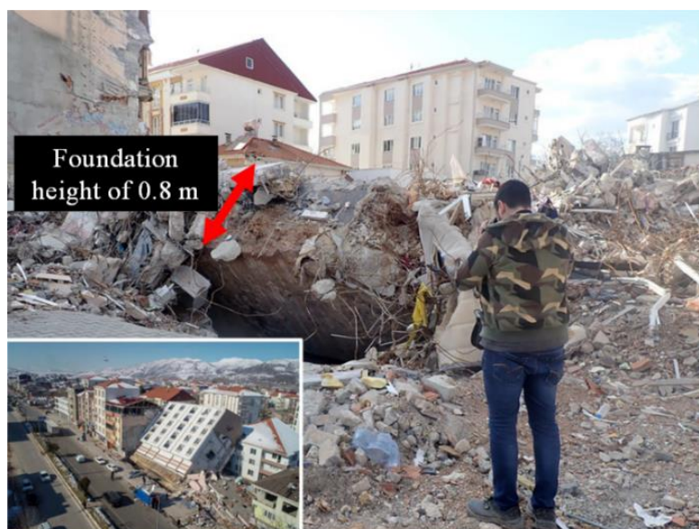
Figure 15. Tilted foundation of demolished building [5]
