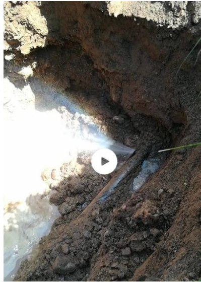
Figure 7. Water loss detection
